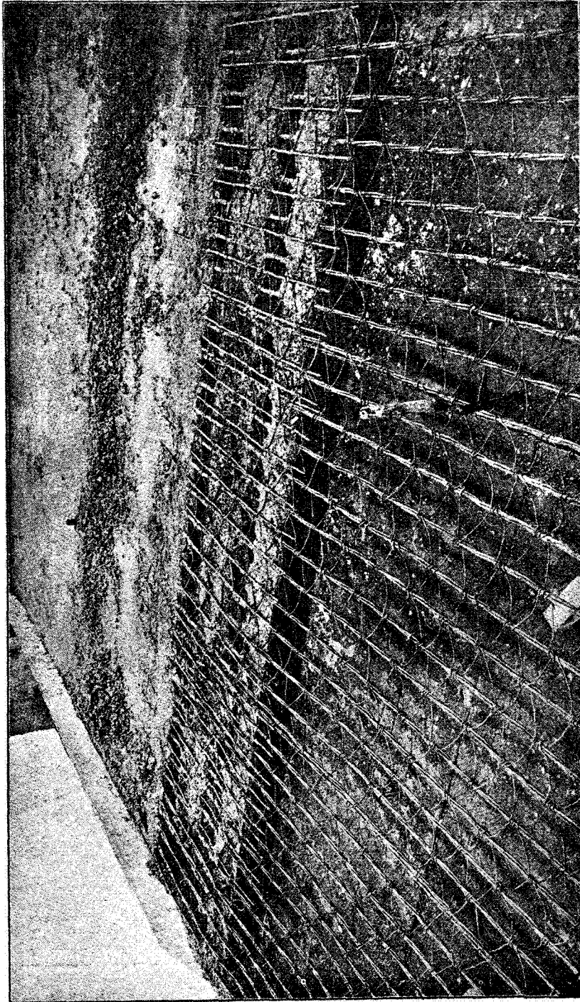
Arrangement of Metal in the Floor. Concrete Partially in Place on the 5-Foot Span. 8-Foot Span in the Foreground.
