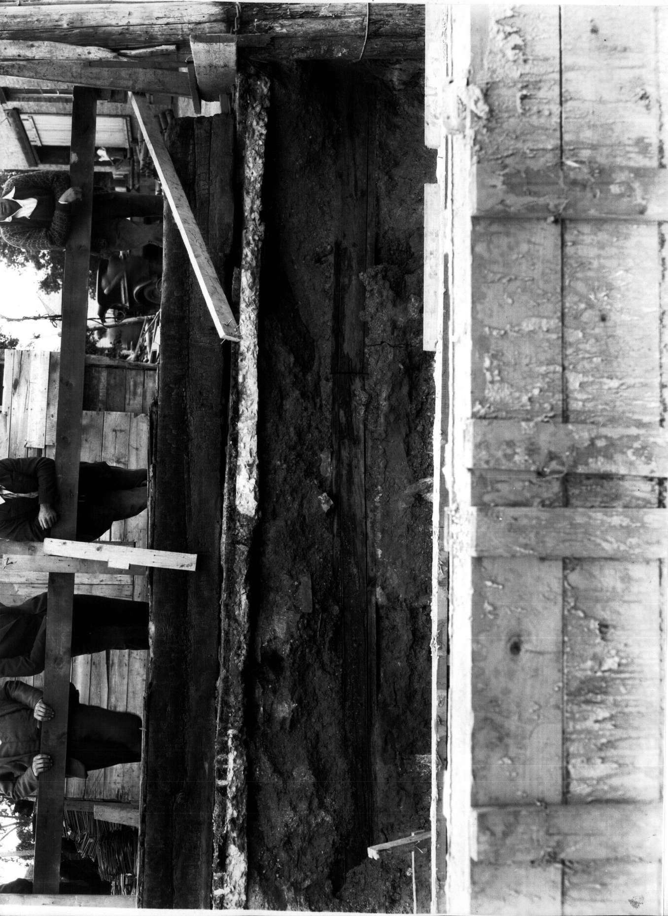
No. 33 Photograph of demolished south wall of Corona Hotel after the fire, showing wooden conduit box. (Plaintiffs' Exhibit)
