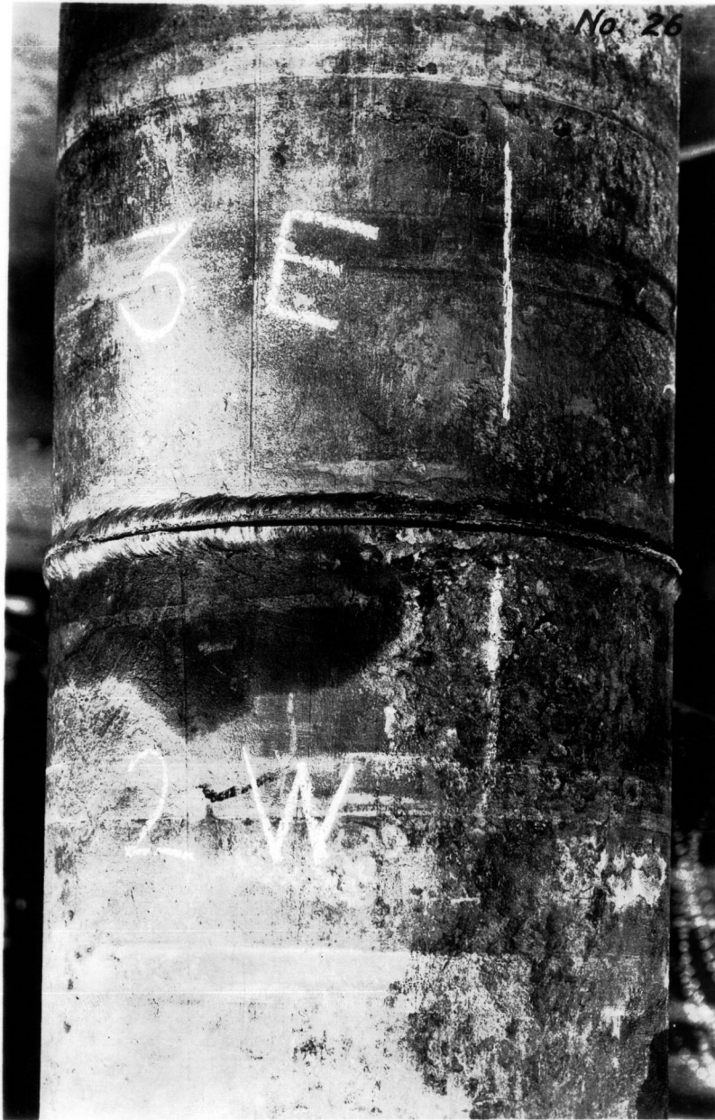
No. 72 Photograph of side view of broken weld (Exhibit 42). (Plaintiffs' Exhibit)
